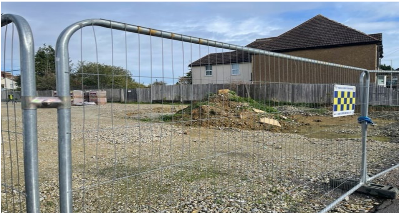
Figure 3: Photo showing the flank elevation of the dwelling. The adjacent car park (under construction) in the foreground
